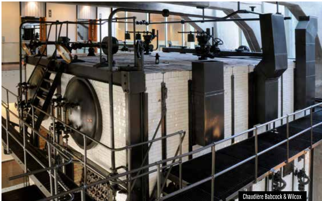
Chaudière Babcock & Wilcox
